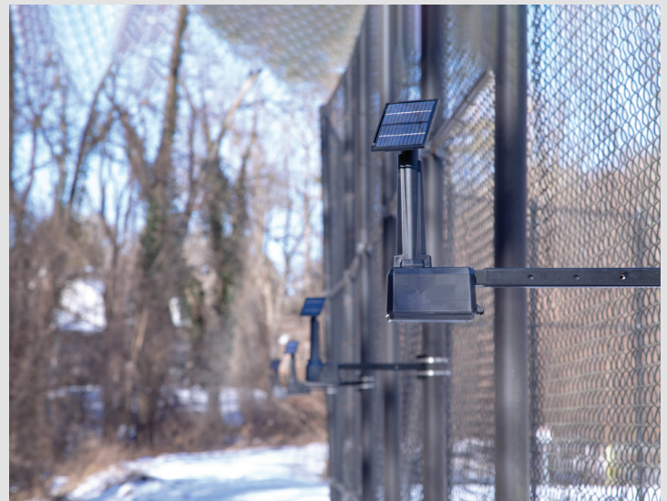
Guardians mounted on fence create a secure perimeter.
